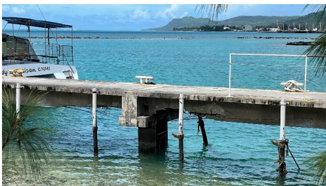
Exhibit D: Exposed rebar on gangway
